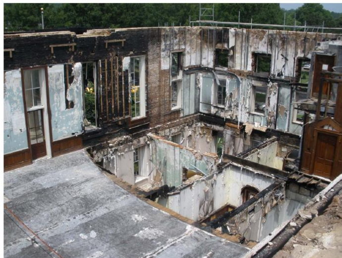
Post Fire Image Chatham County Courthouse
